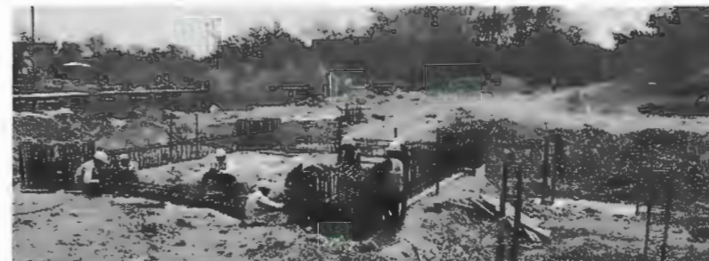
By Product Silo back filling work 90% done. Plinth beam steel binding work under progress.
